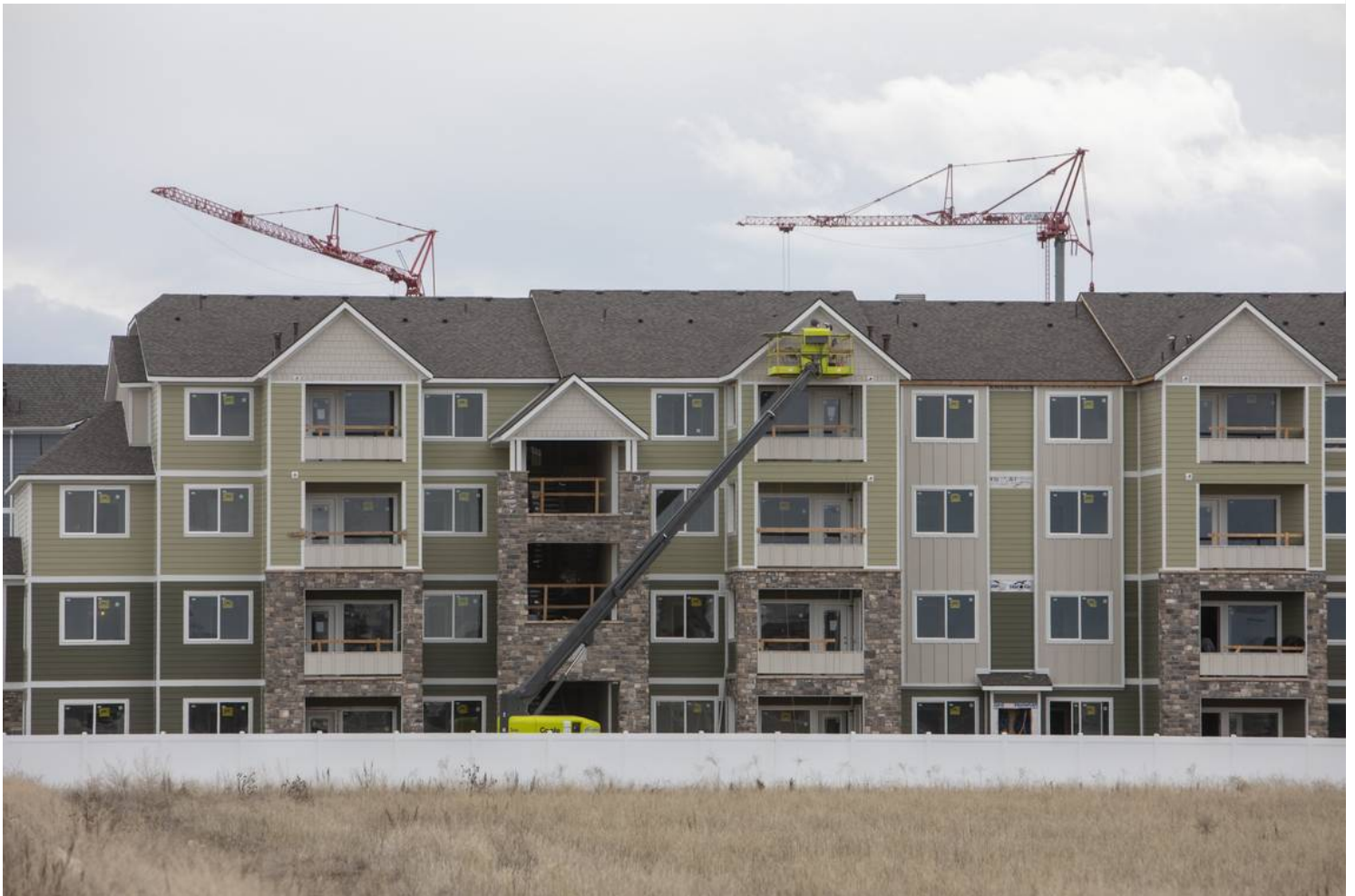
The Regency at River Valley Apartments are going up on Records Avenue near The Village at Meridian. Katherine Jones KJONES@IDAHOSTATESMAN.COM
